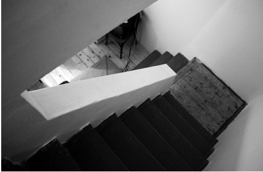
Stairs with rope.
